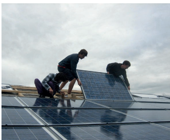
BIPV installation in Switzerland
