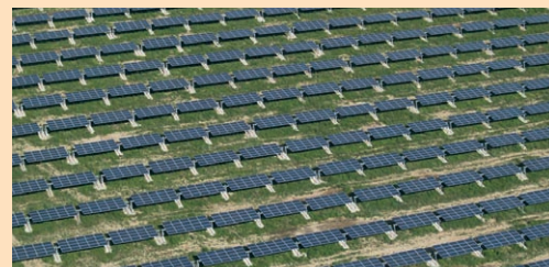
1,1 MW PV Plant in Spain (Courtesy of Edisun Power)
