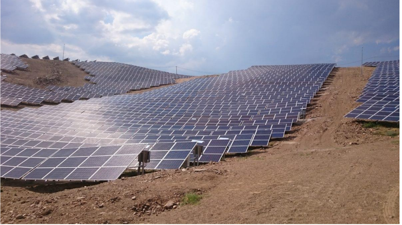
Astronergy modules installed in a 4.3 MW solar park close to city of Cine in western Turkey.
