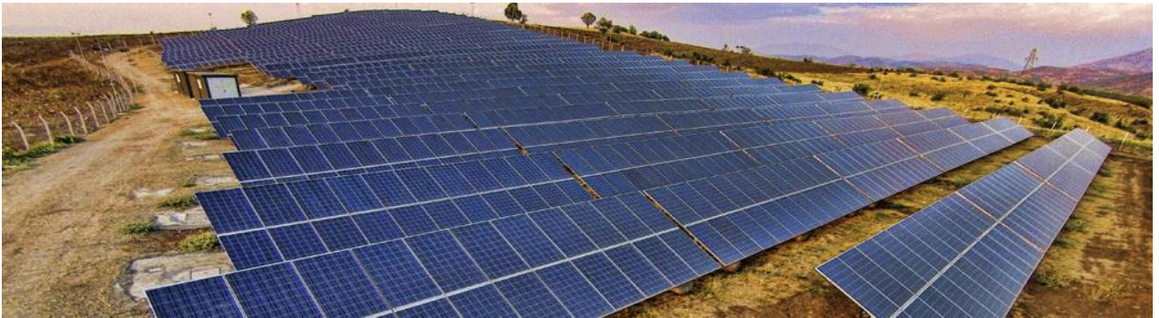
Adiyaman GES is the first PV Plant connected to the MV stage in Turkey.
