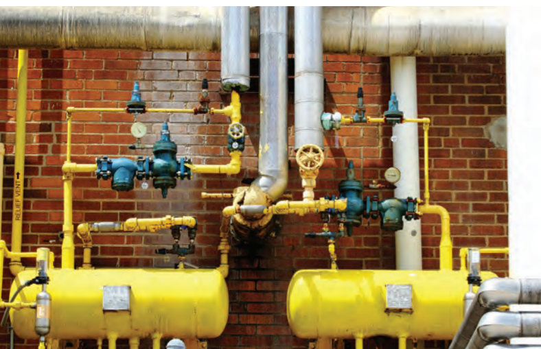
Above: Ammonia refrigeration tanks.
