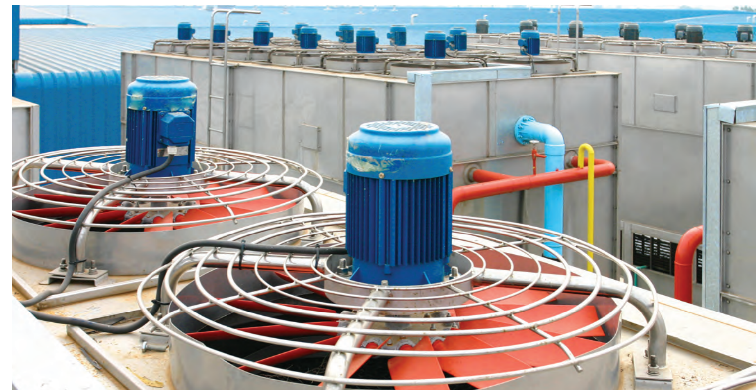
Above: Cooling units on a food processing factory roof.
